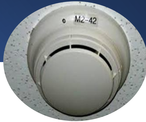
Typical Building Fire Alarm Smoke Detector
