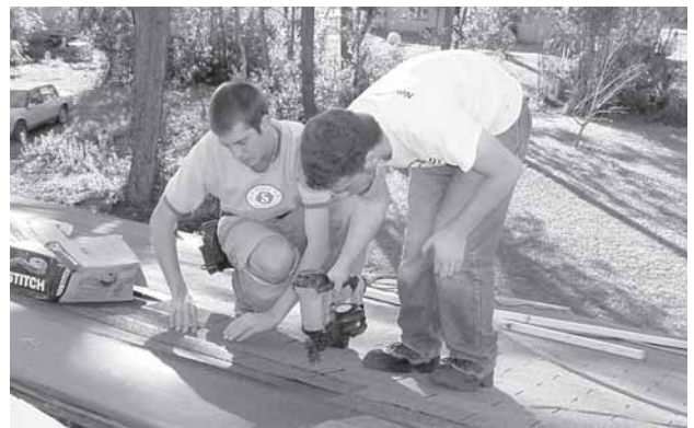
Students from West Chester University and Temple University traveled to Louisiana to replace a roof that was damaged from Hurricane Katrina.
